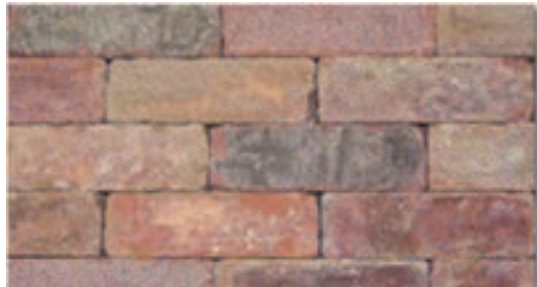
No Mortar Joint (Dry-Stacked)
